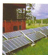
Solar Photo-voltaic Systems
